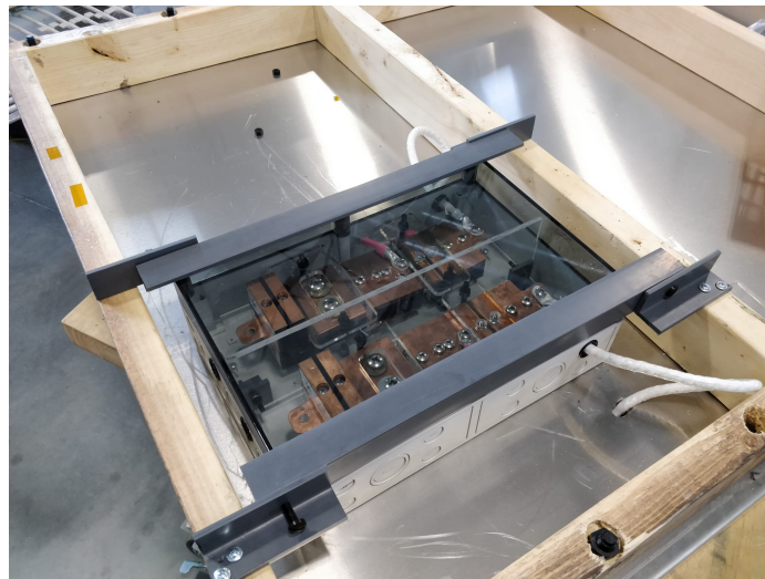
Fig. 5.15: Series compensation capacitors mounted under the primary pad.
